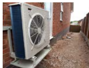
An air source heat pump
