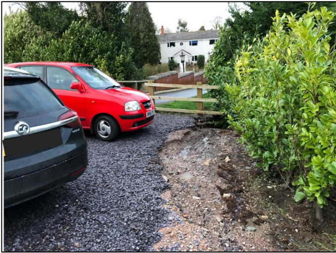
Figure 46: Localised scour caused by overtopping at the discrete low spot (NRW, 2020)
