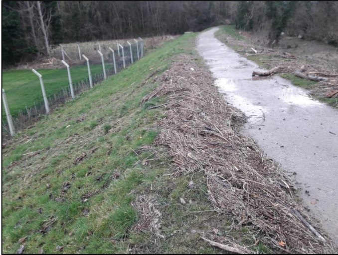
Figure 94: Overtopping location RB STW emb (NRW, 2020)
