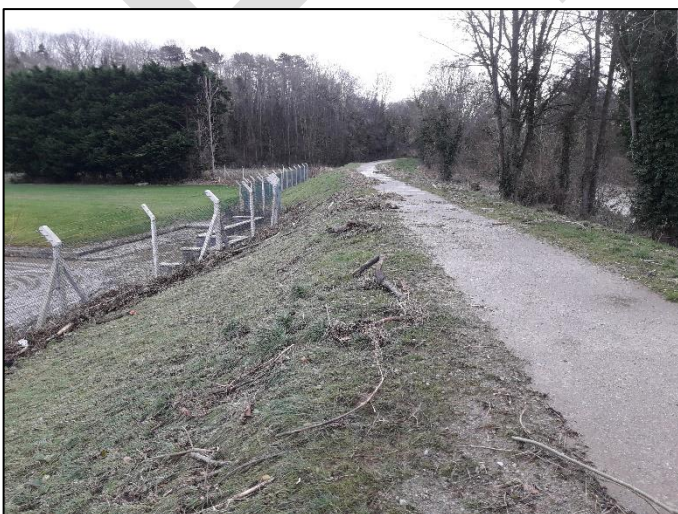
Figure 96: Progression of overtopping RB STW emb (NRW, 2020)
