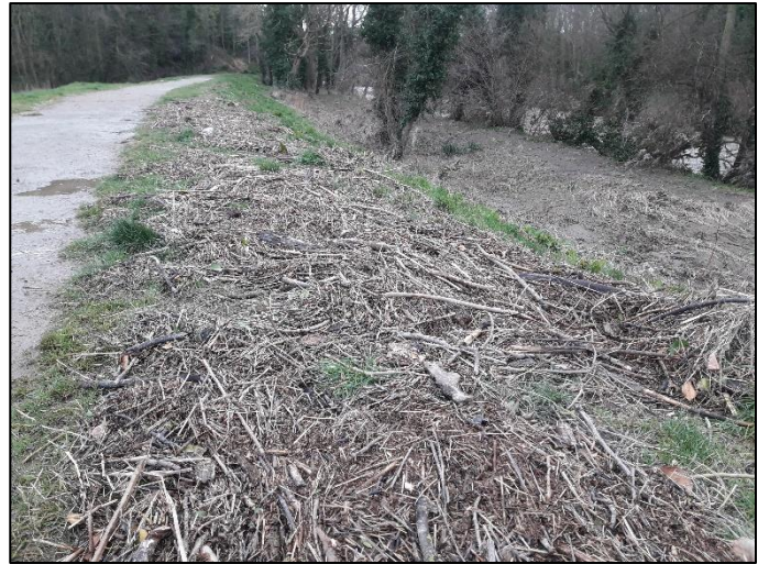
Figure 108: Overtopping location RB STW emb (NRW, 2020)
