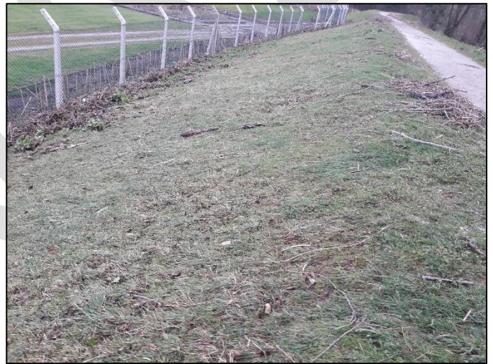
Figure 92: Overtopping location RB STW emb (NRW, 2020)
