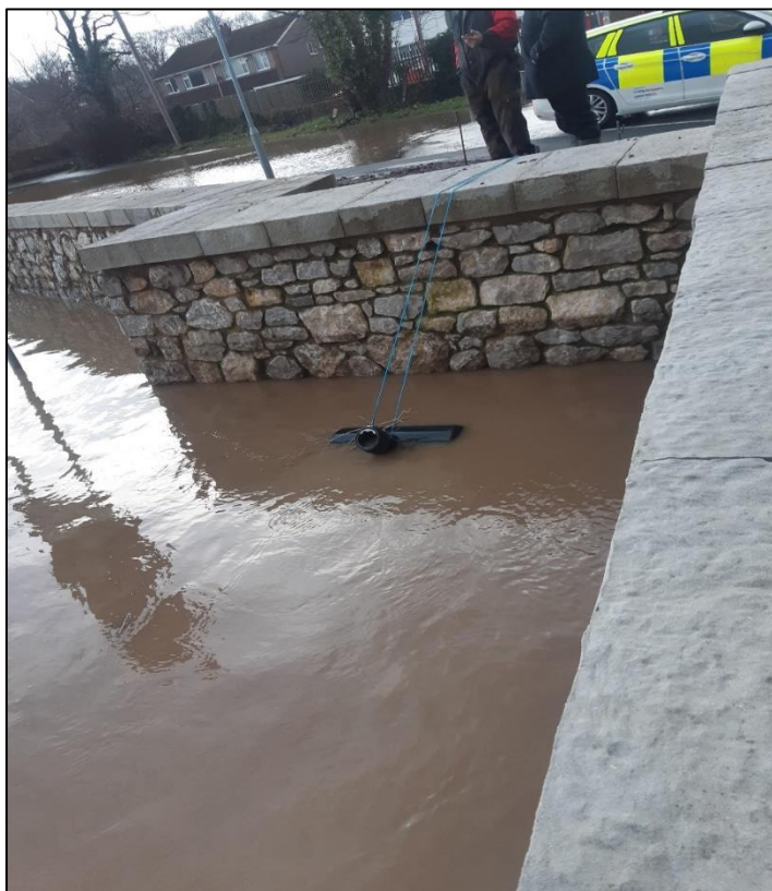
Figure 63: Unauthorised opening of non-return valve (NRW, 2020)
