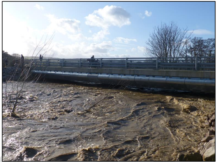
Figure 99: Water levels at SGB (Resident photo)
