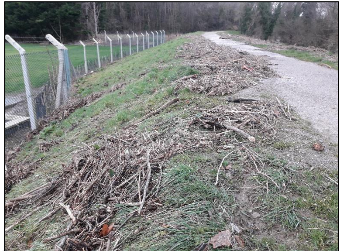
Figure 91: Overtopping location RB STW emb (NRW, 2020)
