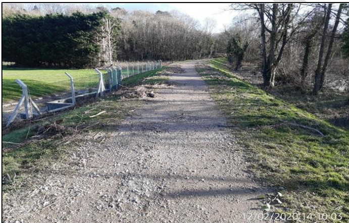
Figure 48: Post Event Inspection RB EMB1800067 (NRW, 2020)
