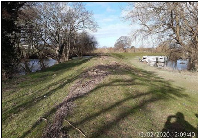
Figure 38: Wrack & debris deposits showing line of overtopping (NRW, 2020)
