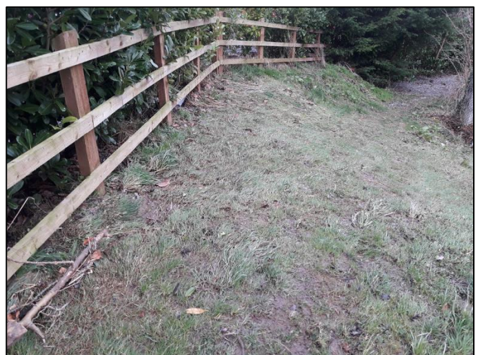
Figure 95: Overtopping location RB STW emb (NRW, 2020)
