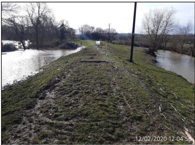
Figure 39: Wrack & debris deposits on the riverside face (NRW, 2020)
