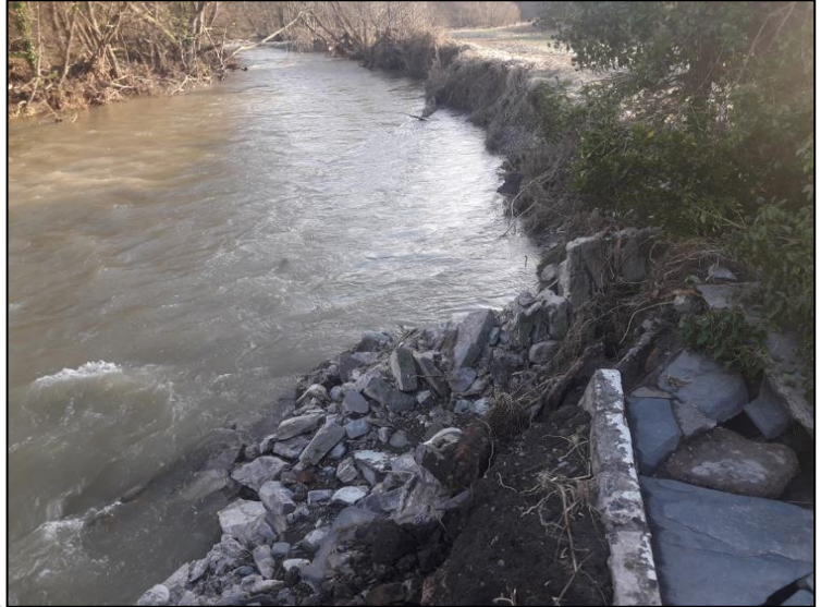
Figure 68: Erosion to private garden, showing historic riverbank revetment (NRW, 2020)
