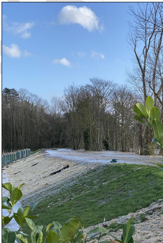
Figure 44: Overtopping of RB EMB1800067 (Resident Photo)
