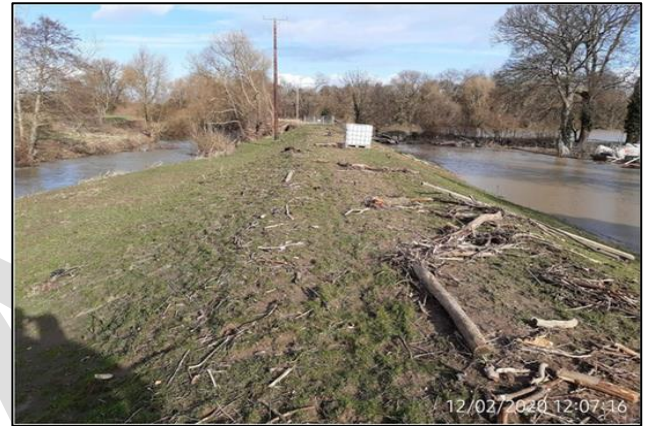
Figure 37: Wrack & debris deposits signifying overtopping location (NRW, 2020)
