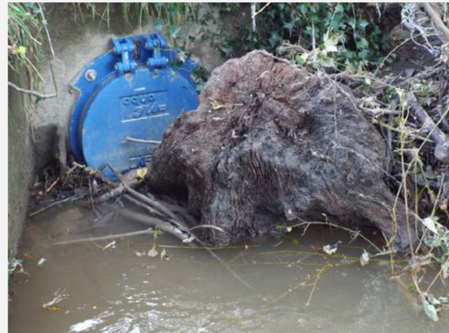
A few days after Storm Babet, a large tree stump was found wedged against the outflow flap valve, probably deposited there during the flood.
